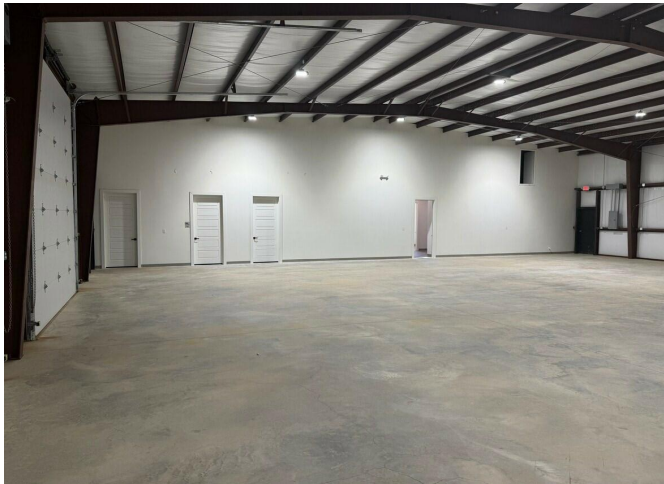
Warehouse — HVAC-conditioned open span with LED lighting
